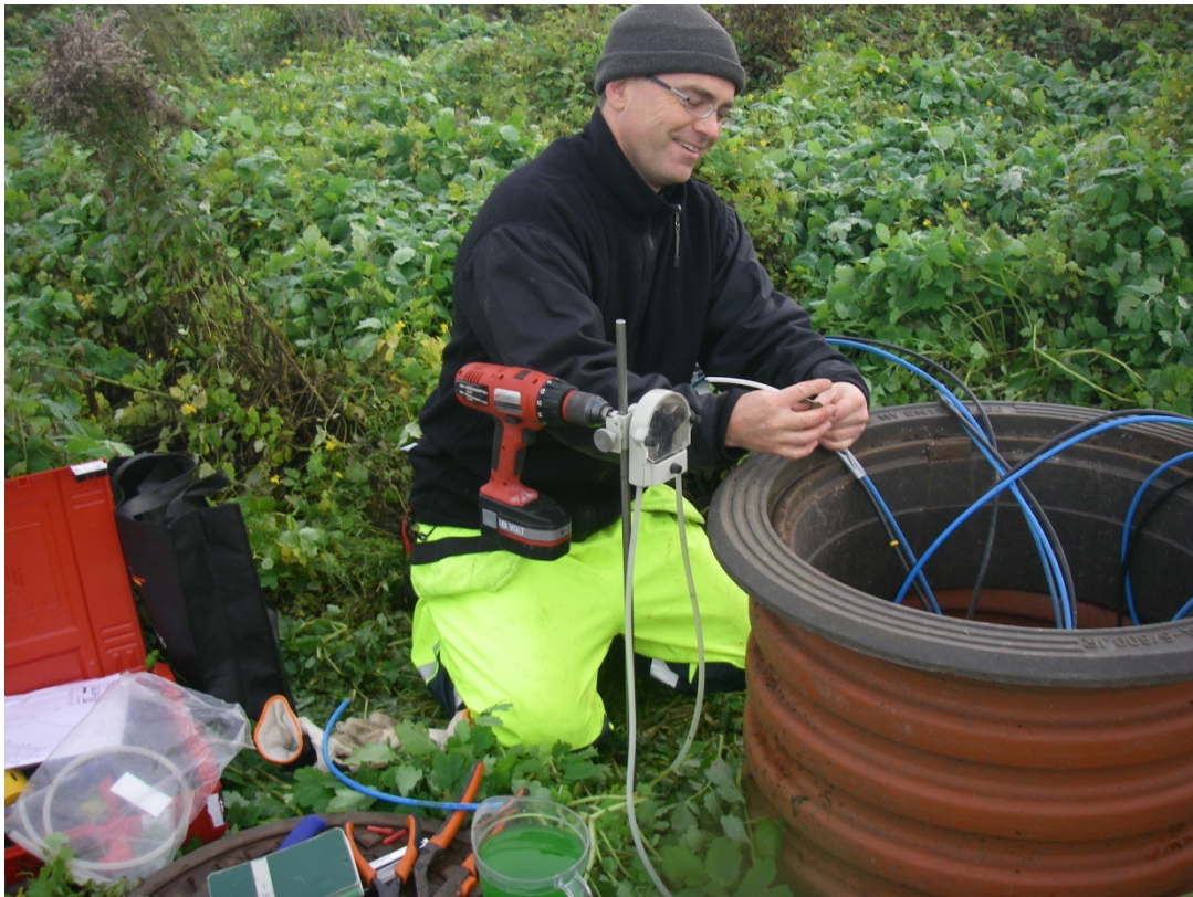
Picture 5 Quality control – Pumping in green water into the lysimeters, in order to check if the system is damage or broken.
