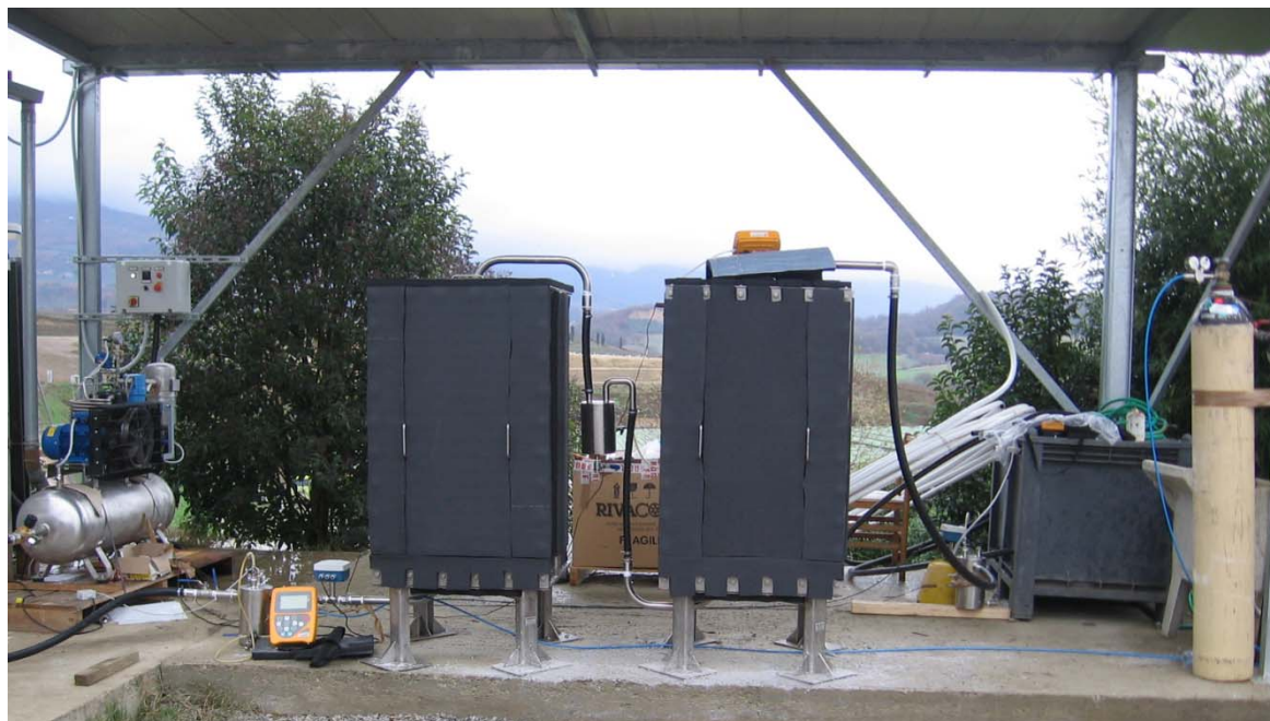
Figure 4b: The Podere Rota pilot plant.
