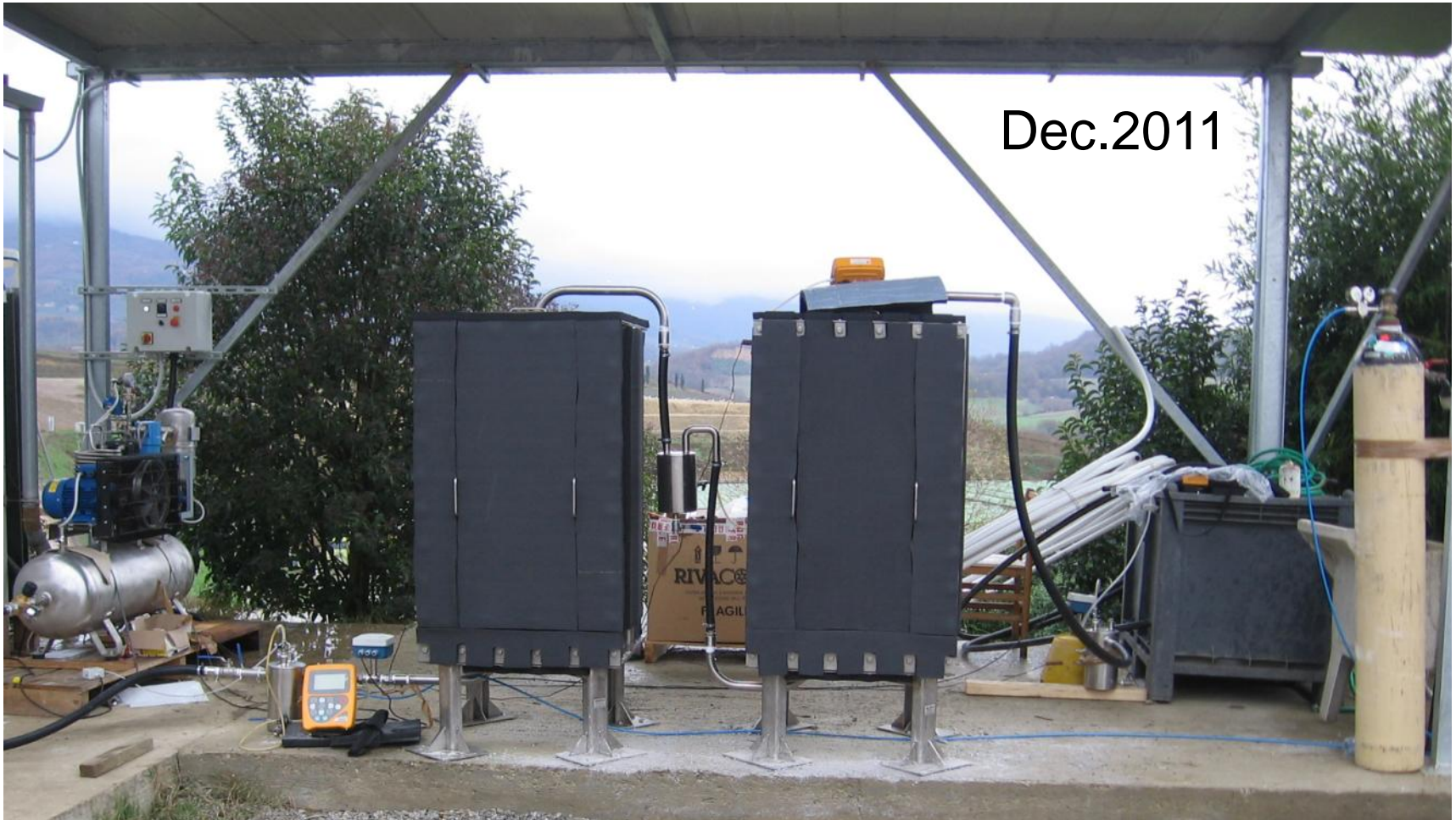
compressor / analyzers / 2 carbonation tanks /
